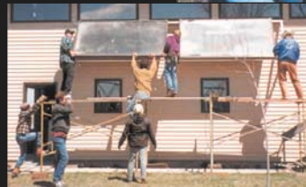
Solar Hot Water
