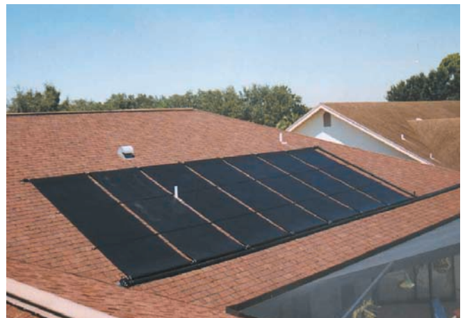
Solar pool panels—roof mounted.
