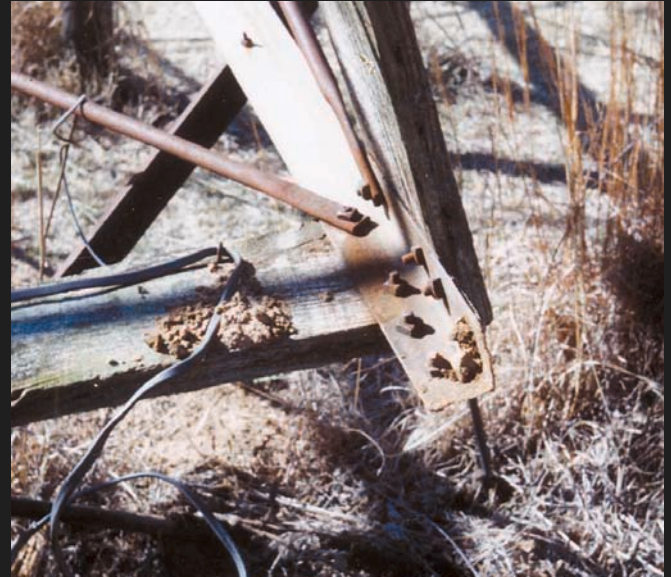
All four tower legs looked like this—completely and squarely rusted off, right at ground level.
