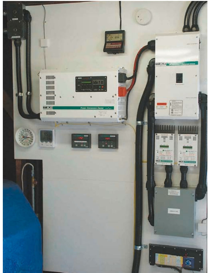
The power panel is installed in the garage.
