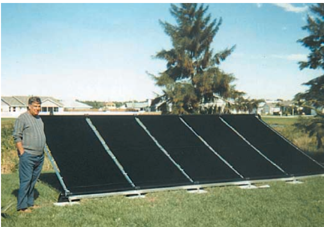
Solar pool panels—ground mounted.
