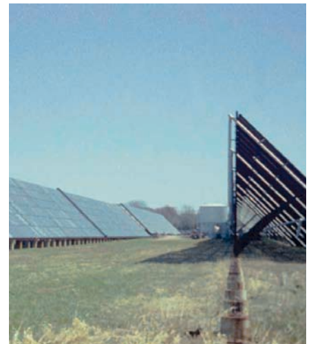
Ground-mounted commercial system.
