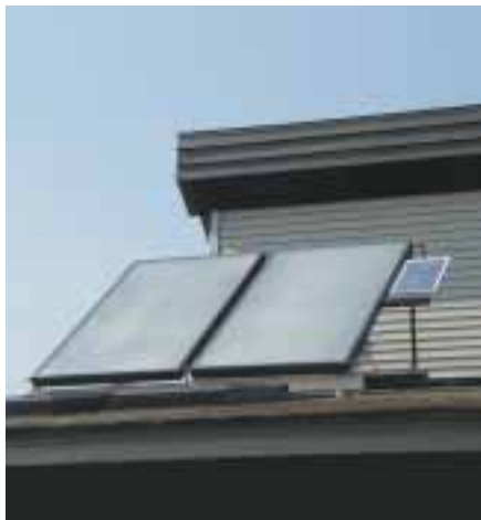
Rack-mounted, PV powered system.
