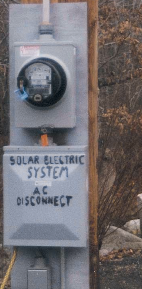
The utility meter and lockable disconnect are the only stationary parts of the system.
